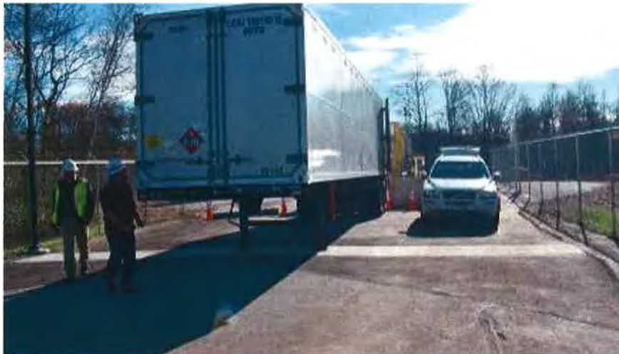
A CNG tank truck was on site to facilitate the system operational testing and operator training.
